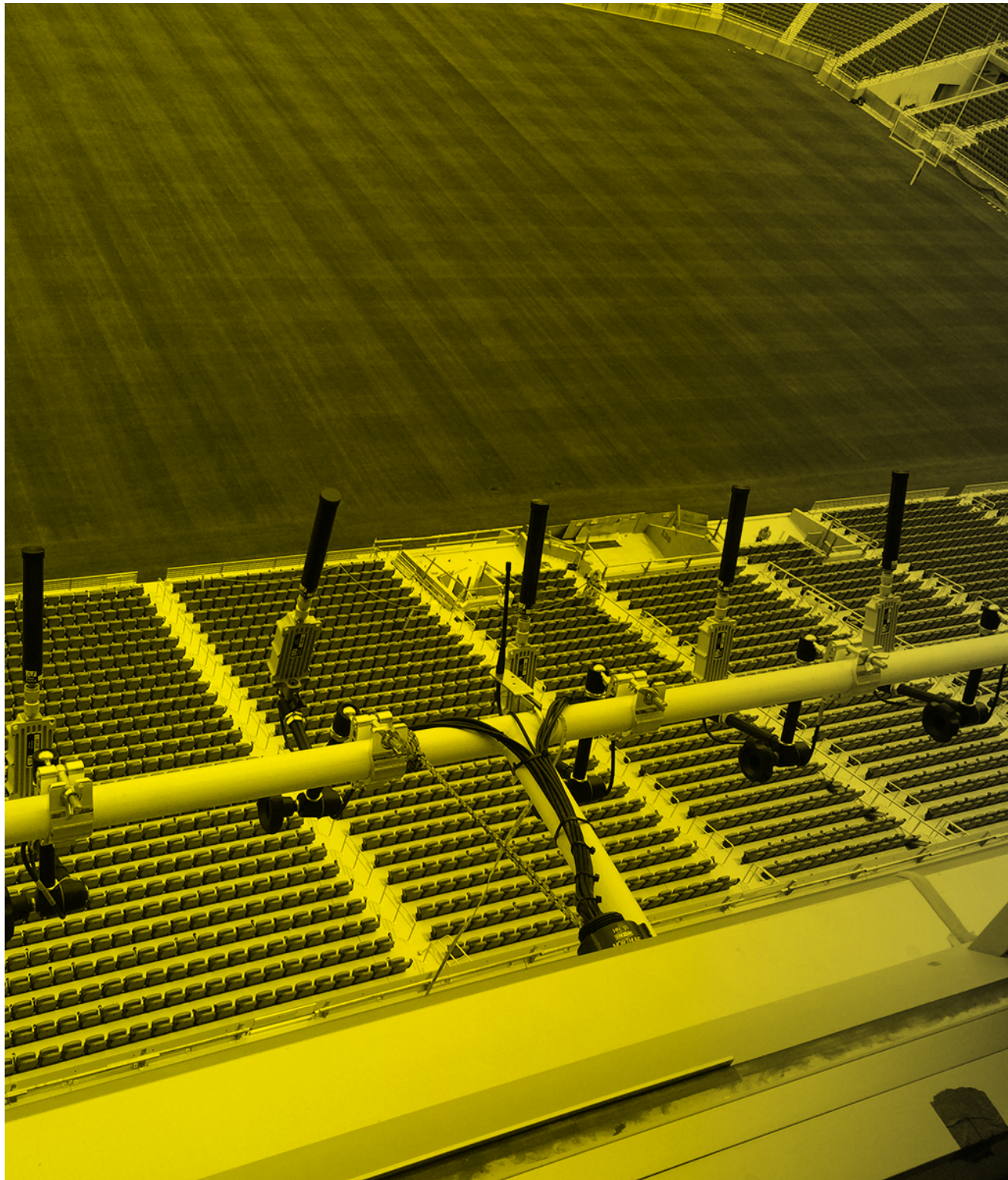
TWO ANTENNA ARRAY
